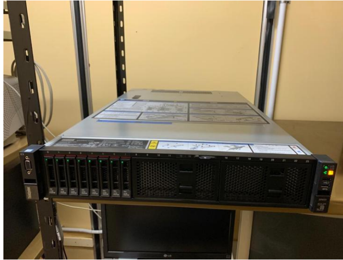
Figure 1: New DAOC server installed and running
